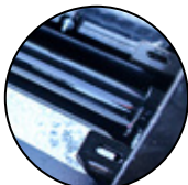
Brackets in tower for pony motor or chain bar
